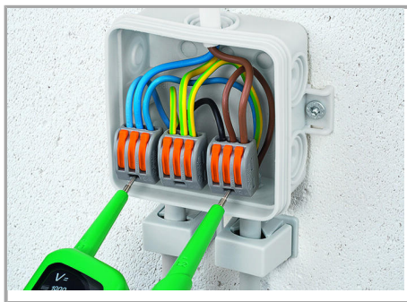
Testing via Profi-LED+ voltage tester (206-806).
